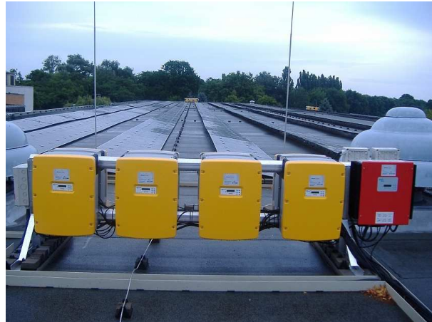
PV system on the roof of a city water treatment plant
