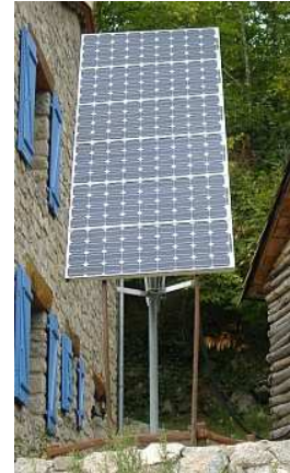
Off-grid solar system, France
