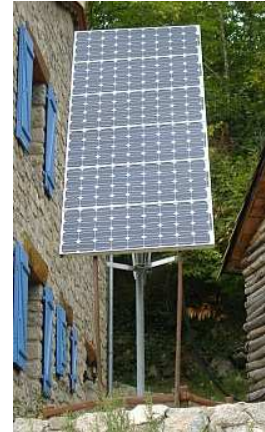
Off-grid solar system, France
