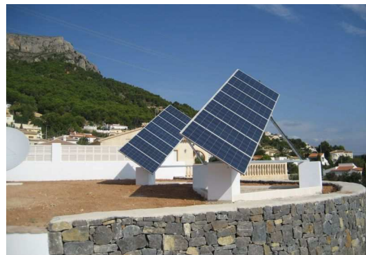
Off-grid solar system in Spain Photo: www-solonet.net
