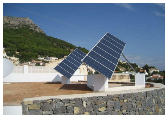
Off-grid solar system in Spain Photo: www-solonet.net
