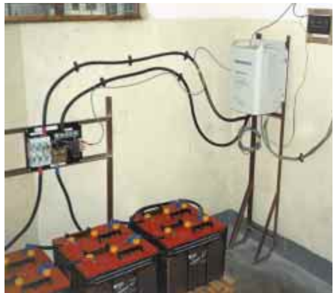
Above: The battery / inverter system..
