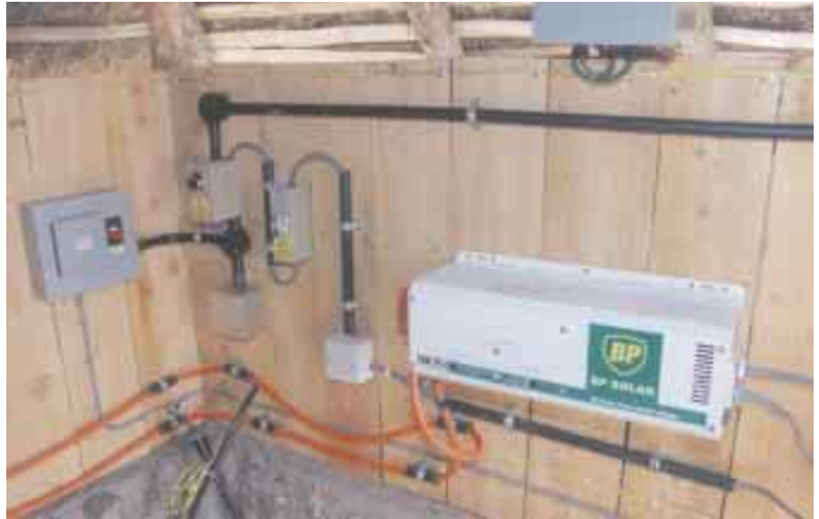
The temporary Trace DR1524 inverter in the battery hut.
